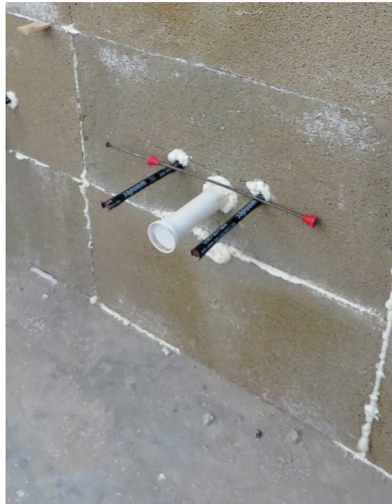
Figure 17: Mechanical items installed in Bautex Wall
